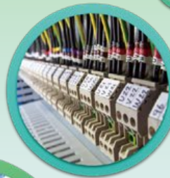
High-Density Branch Circuits Monitoring
